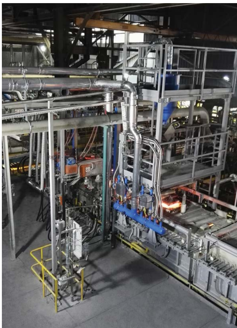
Colouring forehearth installation.
