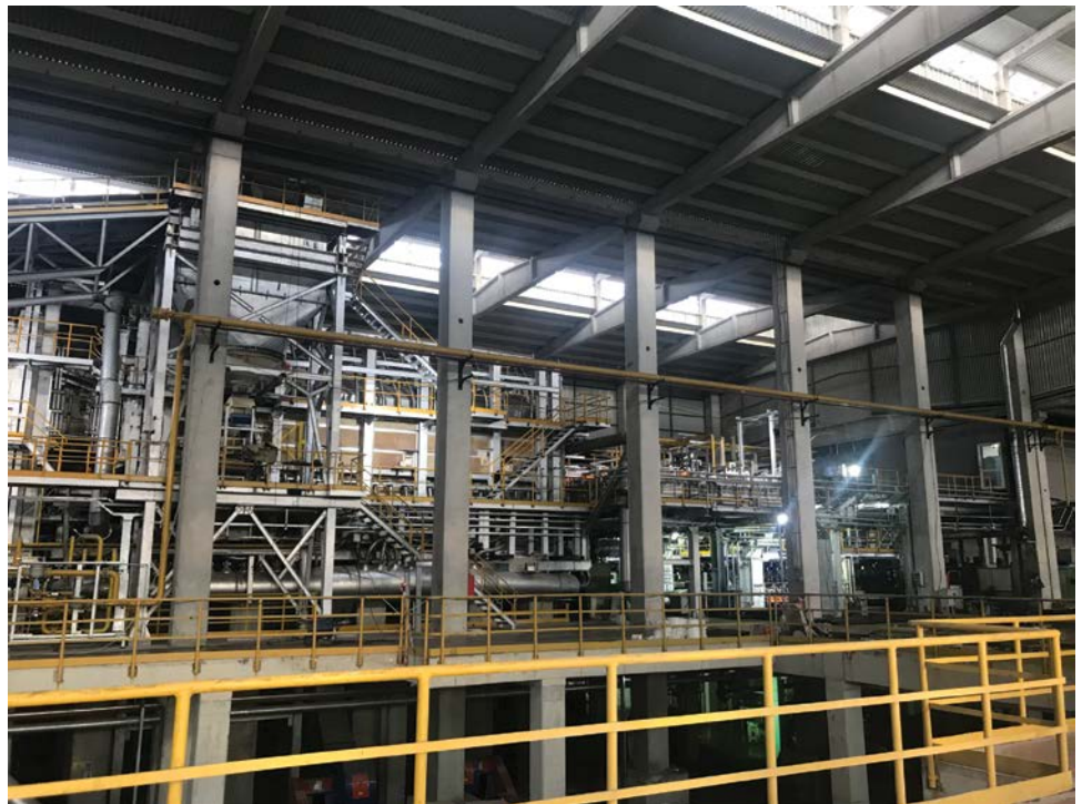
A 300 tonnes/day Falorni regenerative furnace.
